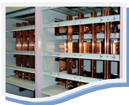
Systems are constructed to meet up to 80kA fault rating (ASTA certified).
